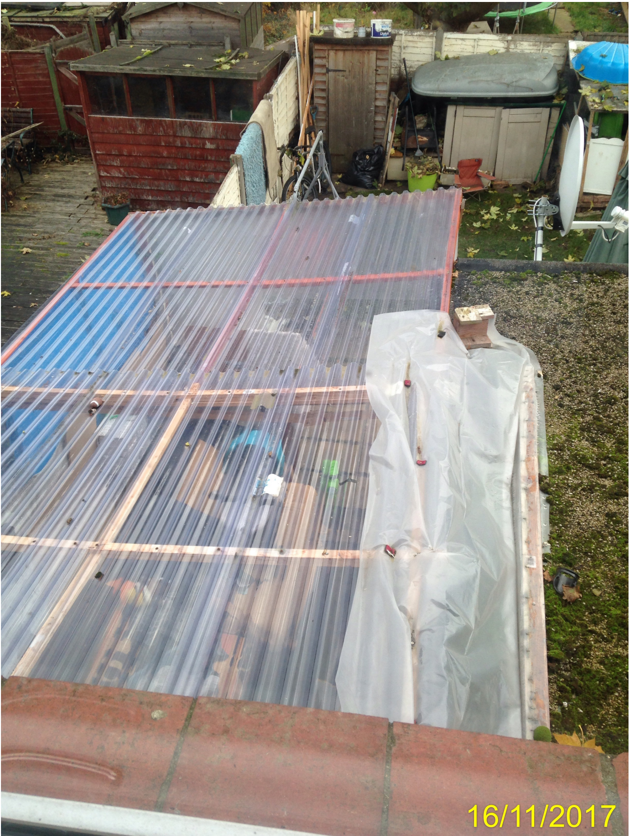
View of corrugated roof of unlawful extension.
